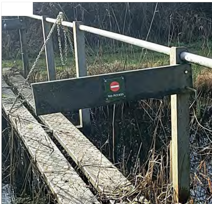
4: Blocked access to vulnerable areas of the site
